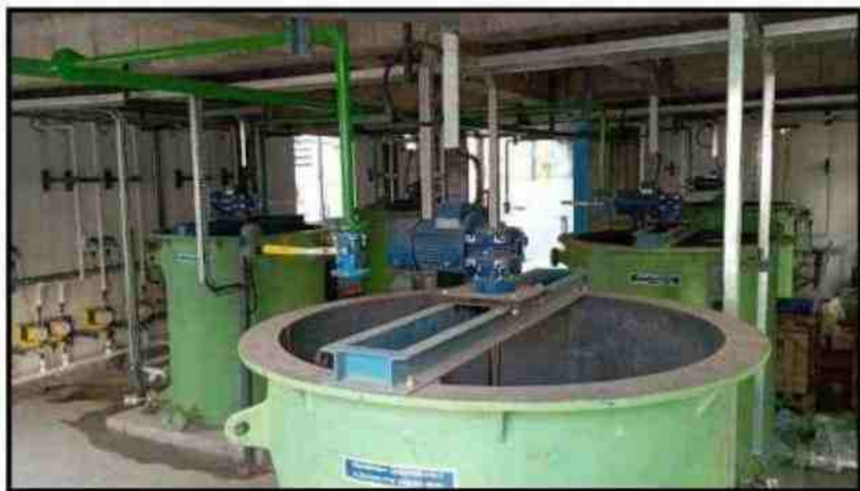
CHEMICAL DOSING SYSTEM, PSF & ACF
